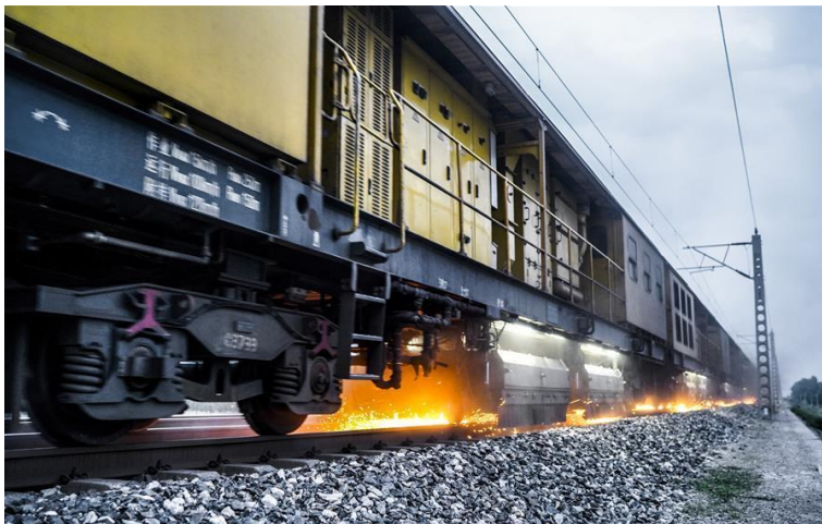
Figure 5: Rail grinding machine works on the rails of Tianjin-Bazhou railway in North China's Tianjin, June 9, 2020
