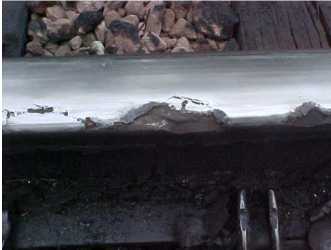
Figure 9: Example 1 of RCF (shells defects)
