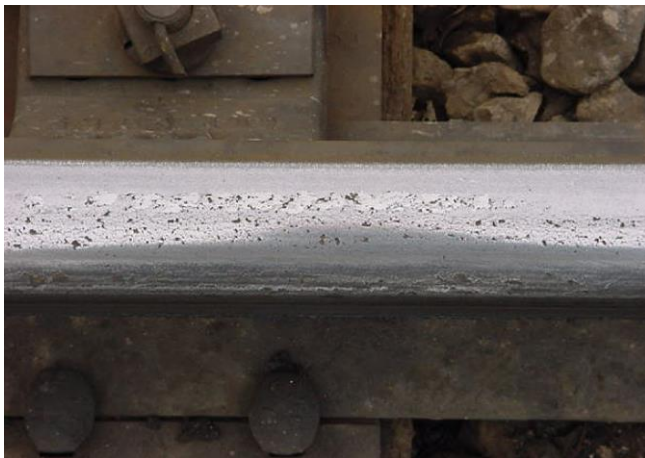
Figure 10: Example 2 of RCF (flaking defects)
