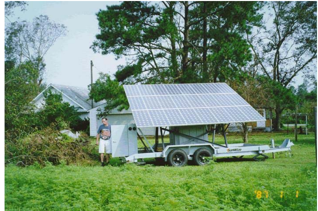
Figure 2. FEMA 1,800 Wp Trailer
