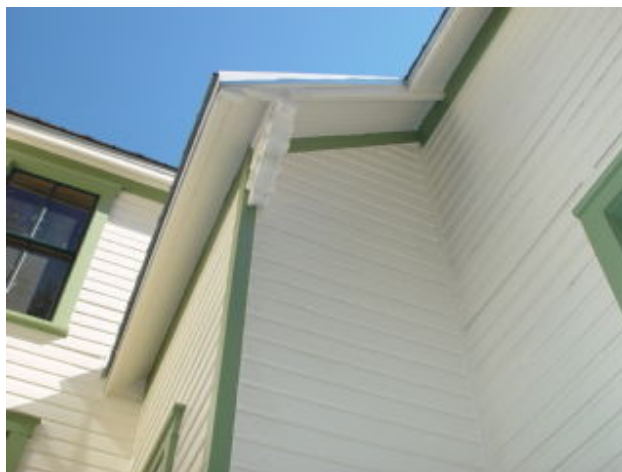
Figure 2 - Solid soffits allow minimal attic ventilation
