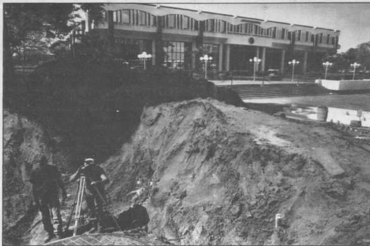
Workers survey an area near the Reflecting Pond, which has been dug up during the installation of the new filtration system and new fountain.
