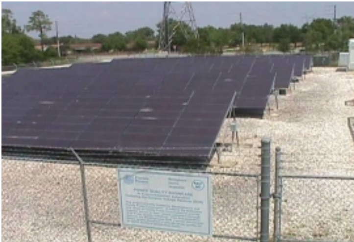
Figure 1. Solar Progress photovoltaic array.
