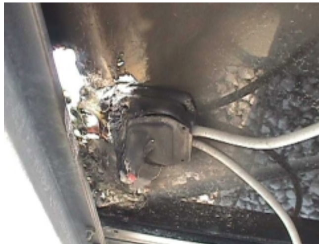
Figure 4. Damage to the module junction box.
