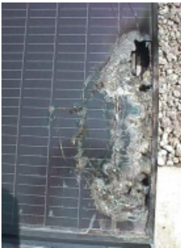
Figure 3. Damage to the module surface.
