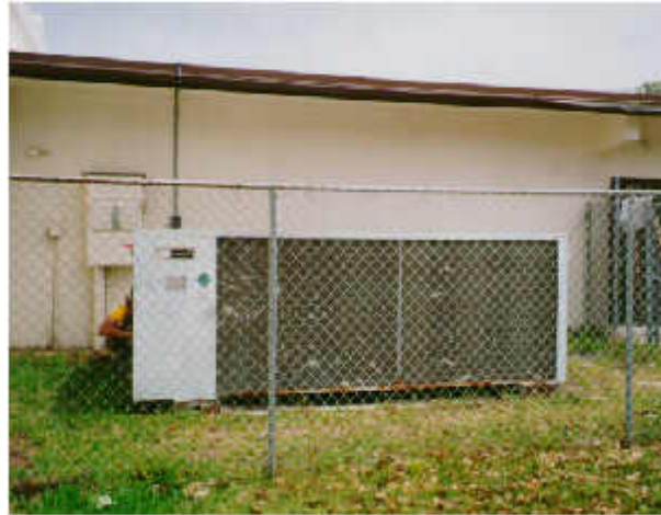
Figure 3. Forty-ton air cooled liquid chiller.
