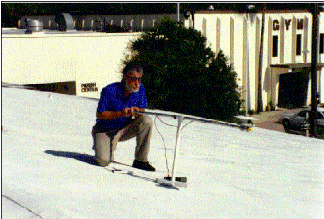
Figure 11. Pyranometer is used to measure roof reflectance one year after initial treatment.
