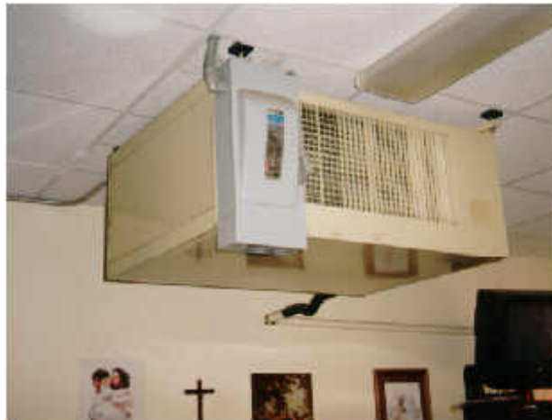
Figure 4. Ceiling mounted classroom air handler. Above acoustic tiles is R-19 insulation. Chilled water lines are located in roof plenum above insulation.
