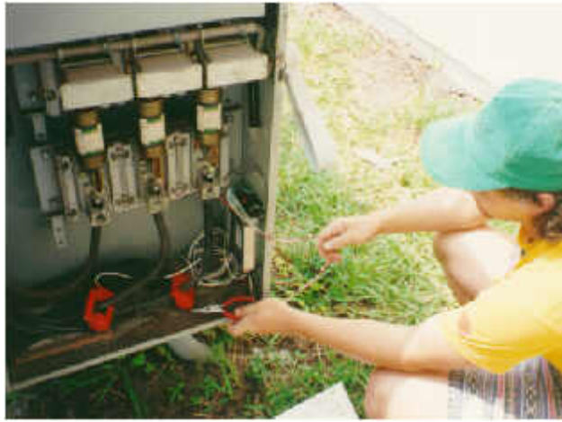
Figure 5. Stephen Barkaszi installs watt-hour transducers on the facility chiller to record electrical consumption.
