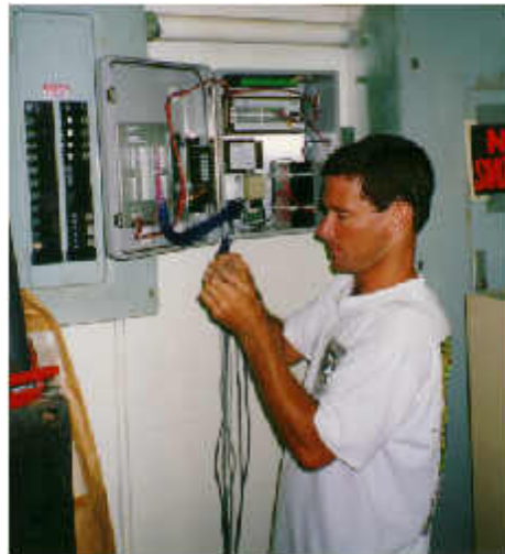
Figure 6. John Sherwin wires in data logger to collect 15-minute data on weather, building thermal conditions, and cooling system electric power.
