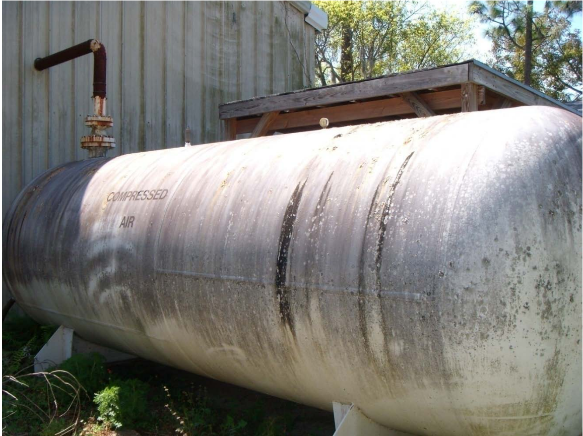
Figure A.6: Five-Thousand Gallon Compressed Air Storage Tank
