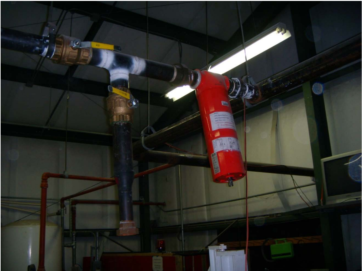
Figure A.5: Three Inch Diameter, Black Iron Supply Line
